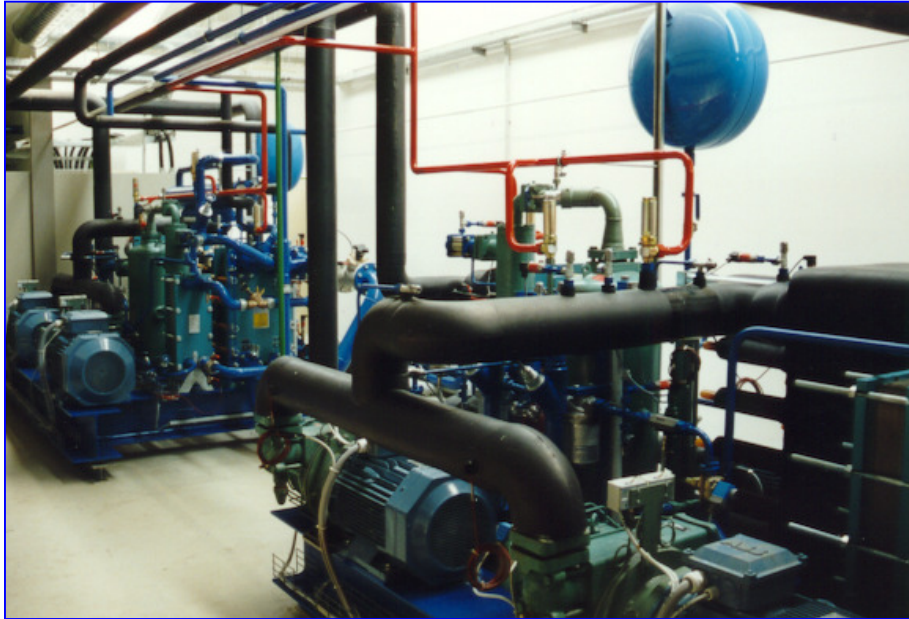
Engine room of an indirect NH 3 system in a hypermarket
